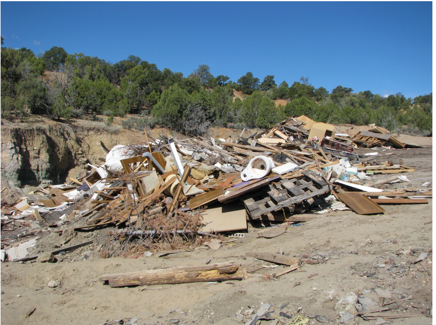
The construction and demolition waste cell. Just a reminder to cover this material once every calendar month
